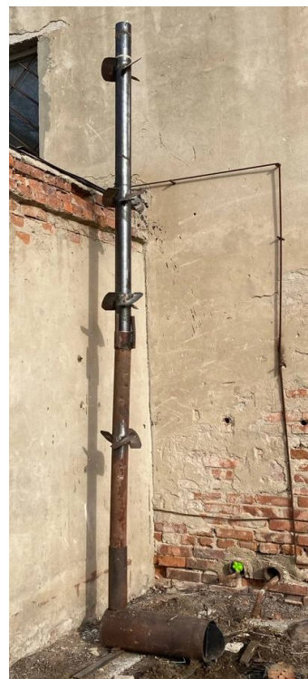
Fig. 2. Chimney with installed vane swirlers
