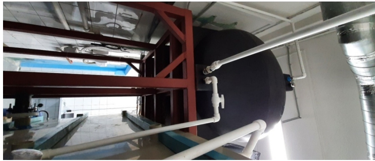
Fig. 3. Unit (water accumulation container) for water treatment
